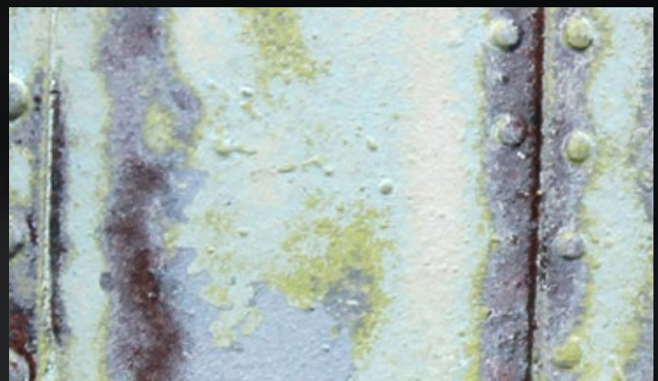
close up of the peeling white paint
